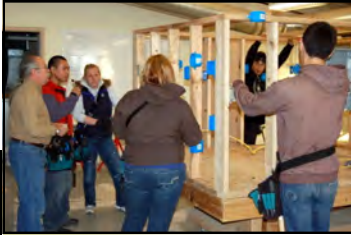
Above: Students in Electrical Level 1 practicing wall socket installation under the supervision of Instructor Steve Reale.
