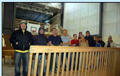
Above: Structural Certificate Students on a piece of the handicapped accessible ramp built for the City of Bethel's Log Cabin.
