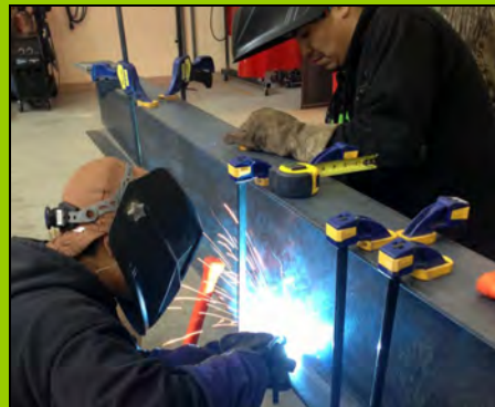
Above: The students building a footbridge for the Yuut Elitnaurviat Campus. This allows them to practice techniques they will need to build boardwalks in their villages.
